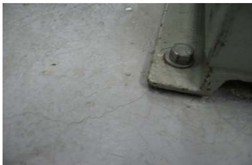
Figure 2. Crack at Control Panel
