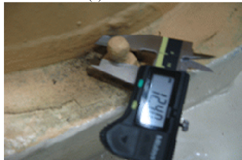
(b) Steel Corrosion
